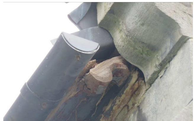
Above : Timber decay threatens gutter fixings. This is the south chapel gutter, similar issue to north aisle.
