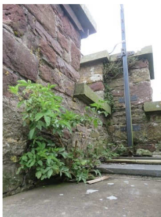
Above : Vegetation growth over vice stair.
