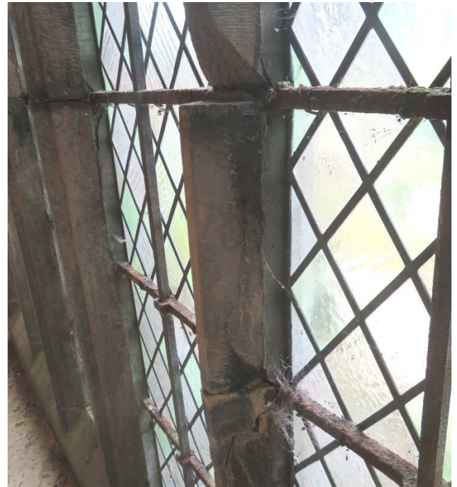
Above : North Aisle, East window. Superficially the glazing is in fair order but the extensive corrosion of metalwork internally, and associated stonework damage threatens stability and is buckling glass in places.
