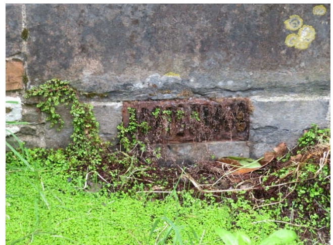
Above : Wall vents rusted up, no longer ventilating beneath the floors.
