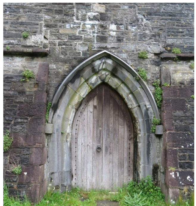
Above : Staining after rain and extensive vegetation growth indicates saturation in the base of the tower. Calcite streaks over the door may also indicate water
