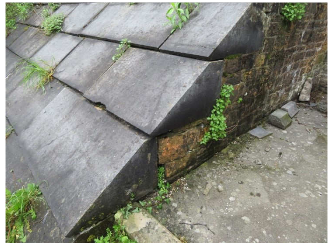
Left : Stone tabling over the Dinefwr vault is very vulnerable to damage from vegetation and washing out of joints.
