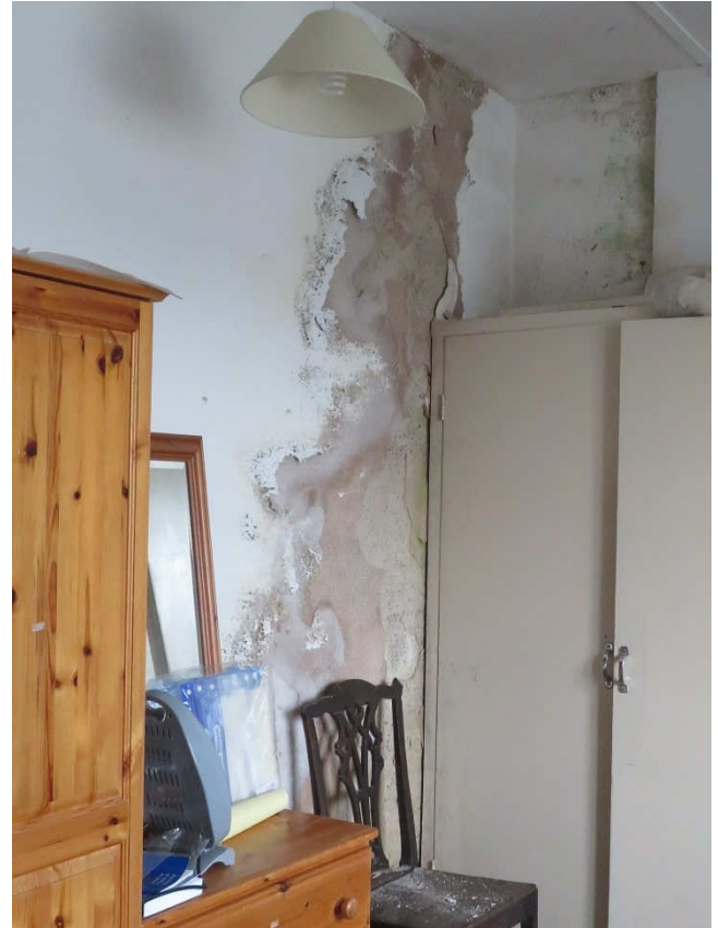
Above : Water damage to plasterwork / decorations in the vestry.
