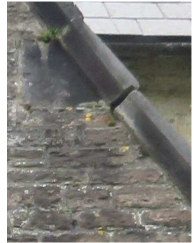
Above : Detail of enlarged open joint to coping stones.
