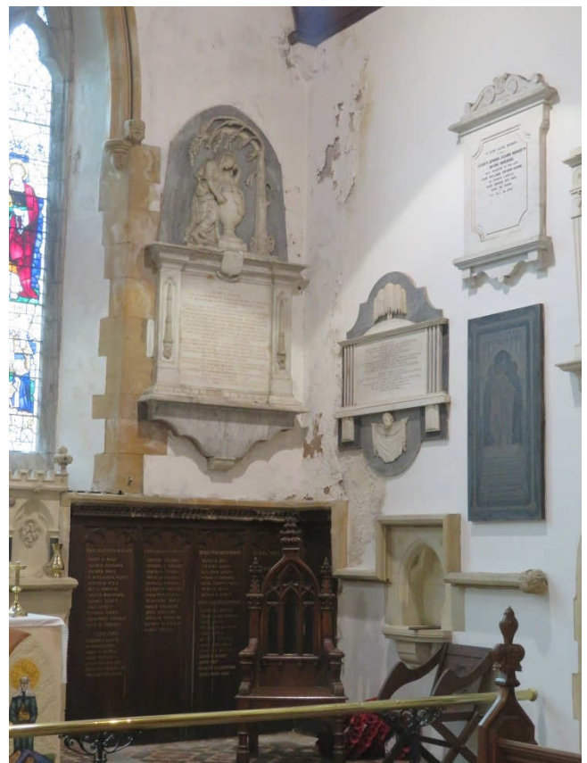
Above : South east corner of chancel : Water ingress damaging plasterwork and decorations, stonework, causing decay to memorial panelling and threatening the wall mounted monuments.
