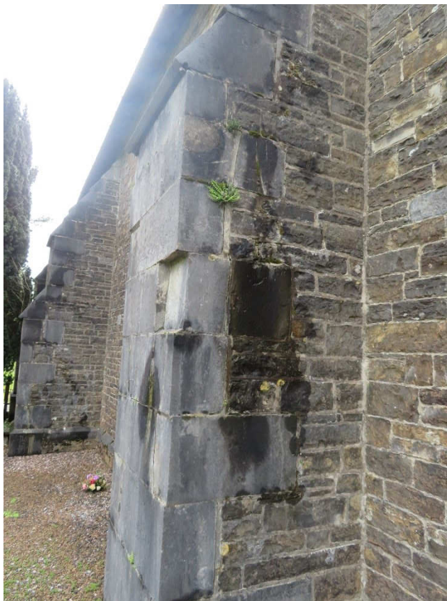
Above : Damaged Carboniferous stonework to buttress, water weeping after rainfall.
