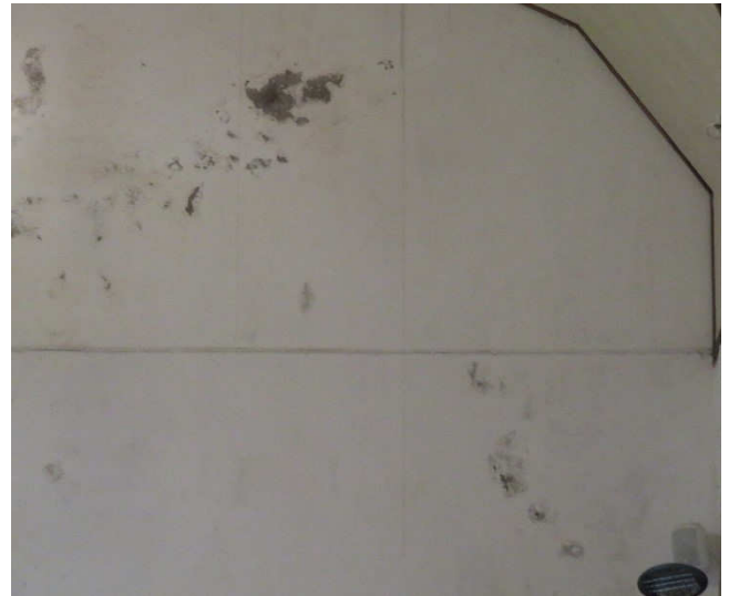
Above : Water damaged decorations and plasterwork to the west nave wall, abutting the tower.
