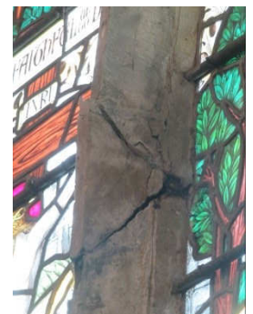
Above : Stone damage, east window (chancel).
