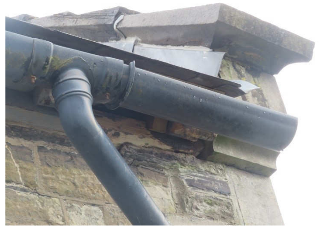
Above : Vestry gutter dropped and overflowing.
