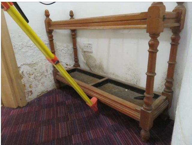
Above : dampness in the WC vestibule and associated condensation / mould growth is occurring in adjacent areas. Further investigation needed.
