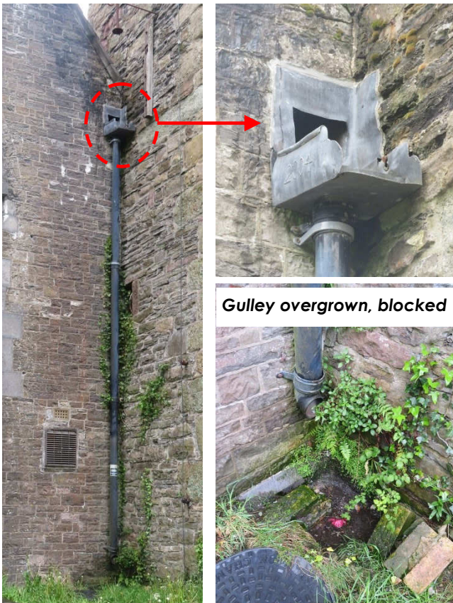
Above : West end. Extensive vegetation growth shows that rainwater goods are not operating fully.
