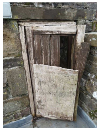
Above : Door in poor condition.
